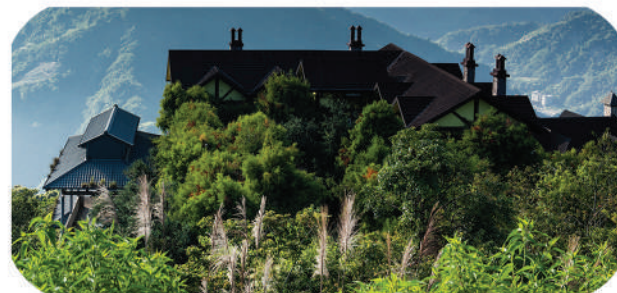
Green PV System for Hotel
